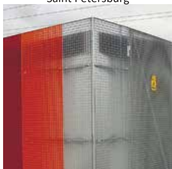
Electrical substation facade protection
